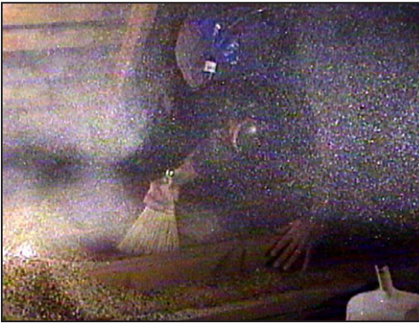
Dust particles generated by the disturbed vermiculite are invisible to the human eye. The scientists at Materials Analytical Services in Suwanee, Ga. have refined the use of Tyntall lighting, which uses special high intensity illumination to scatter light off microscopic particles.
